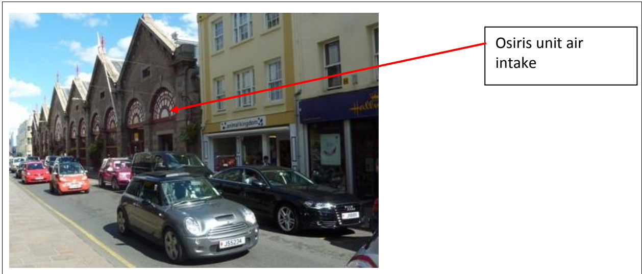
Photograph 2: The Position of the Osiris Unit Ref 2131 at the Central Market, Halkett Place, St Helier
